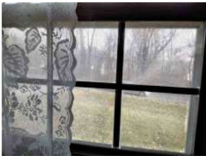
MPR-Cracked window in bedroom 3
