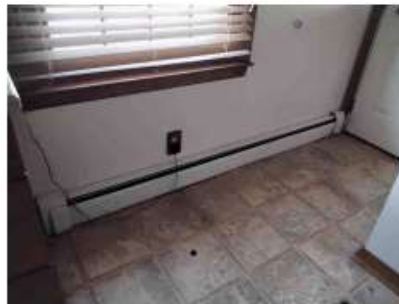
Hot water baseboard heat
