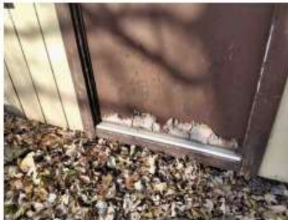
MPR- Chipped and peeling paint/wood deterioration on shed 1 exterior door
