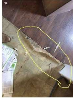
Floor covering trip hazard
