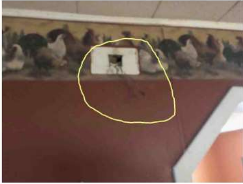
Exposed Electrical wire in the Kitchen
