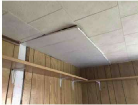
Ceiling in bedroom appears to have been damaged
