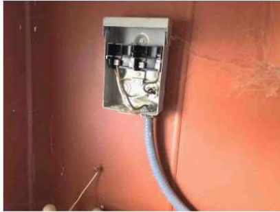
Exposed electrical panel at the hot water heater.
