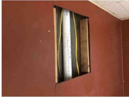
Hole in wall exposing a pipe and wires
