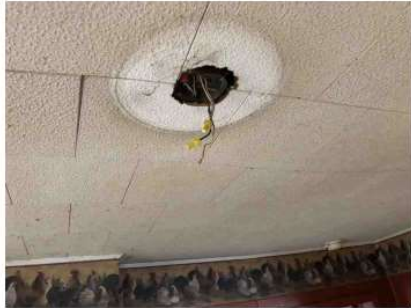
Exposed wires in the kitchen
